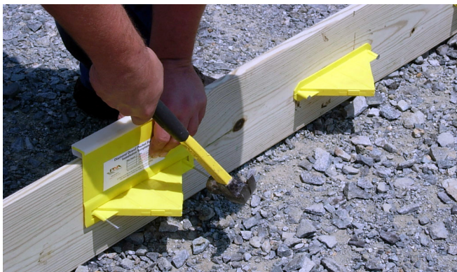
Figure 6. Installation of a diamond plate dowel pocket former [photo courtesy of PNA Construction Technologies].
