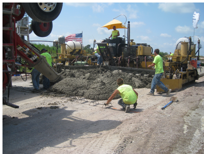
Figure 9. Slipform paving an industrial pavement that includes tapered plate dowel baskets [photo courtesy of PNA Construction Technologies]. Note that the pavement was 8 in. thick and the increased installation tolerances of the tapered plate dowel baskets aided in their placement in front of slipform paving operations, in turn allowing the prepared subgrade to be utilized as a haul road.
